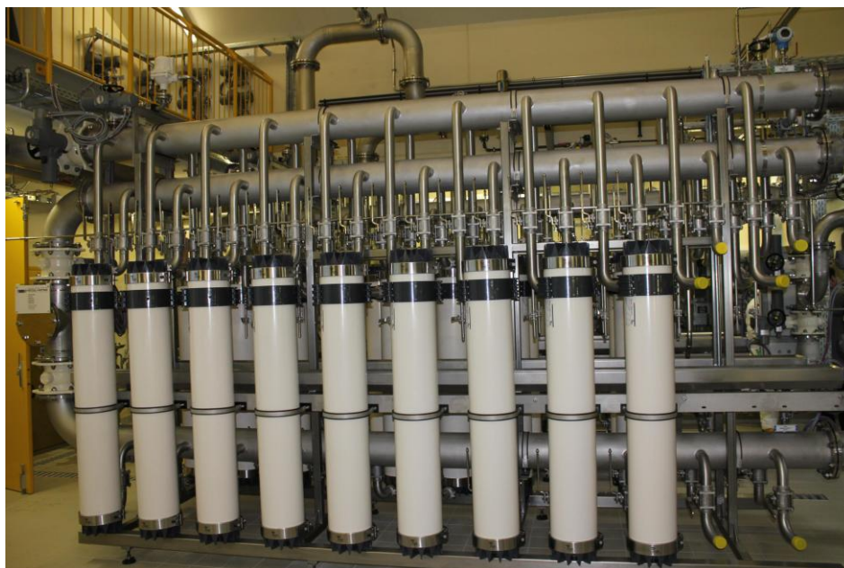
Bildunterschrift: Clean drinking water for the city of Luxembourg thanks to cutting-edge ultrafiltration technology
