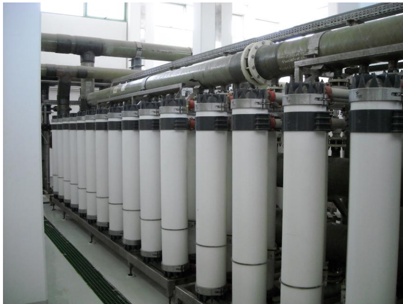
Photo: The ultrafiltration system in Abu Dhabi supplied by inge watertechnologies AG will treat 80,000 m 3 of water a day.
